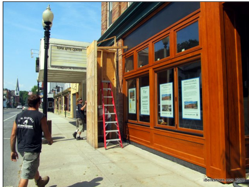
Workers pulled off the protective covering Wednesday afternoon revealing the facade work on the historic building.
